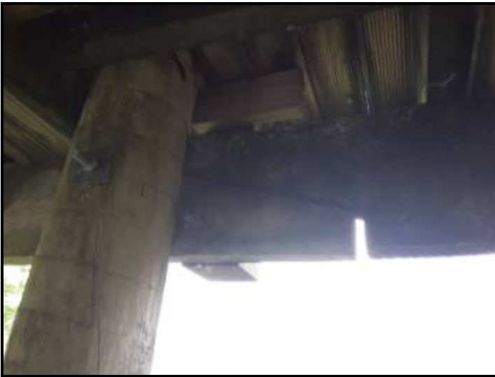
Unprofessional join to beam
