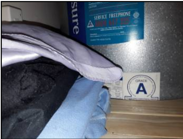
No seismic straps fitted.
