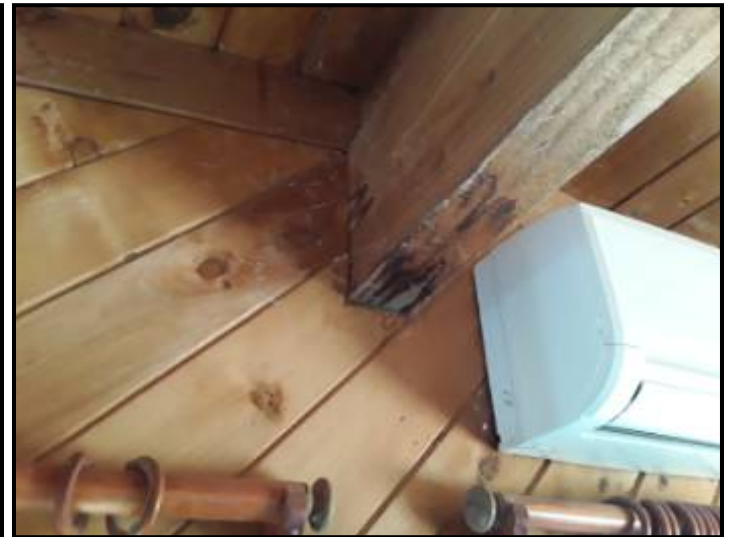
There is signs of water ingress to ridge beam.
