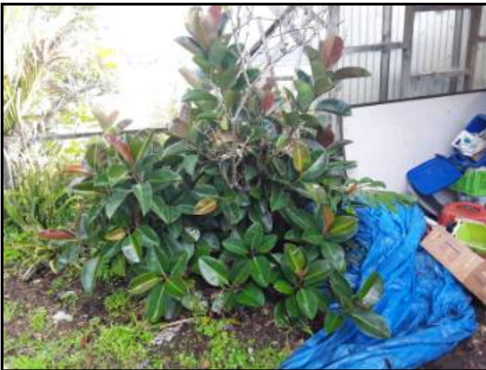
Vegetation too close to house area.
