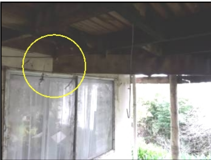
Unprofessional connection here.
