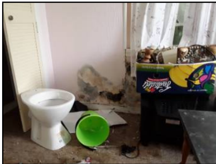
Water ingress has destroyed wall lining.
