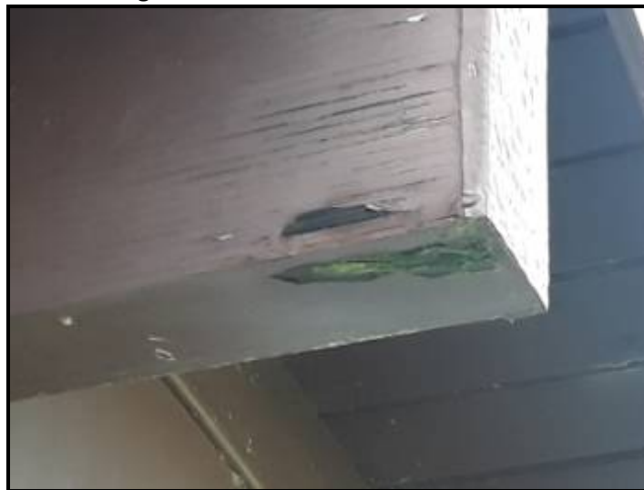
Ridge beam rotting.
