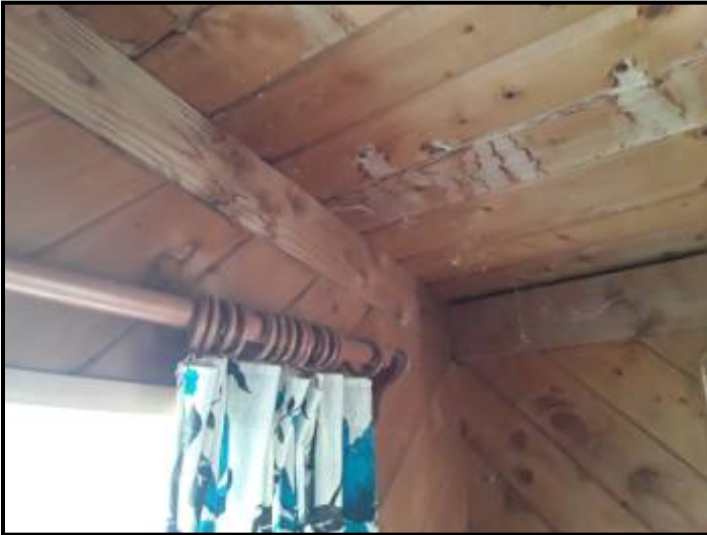
Old water stains. Tested dry here.
