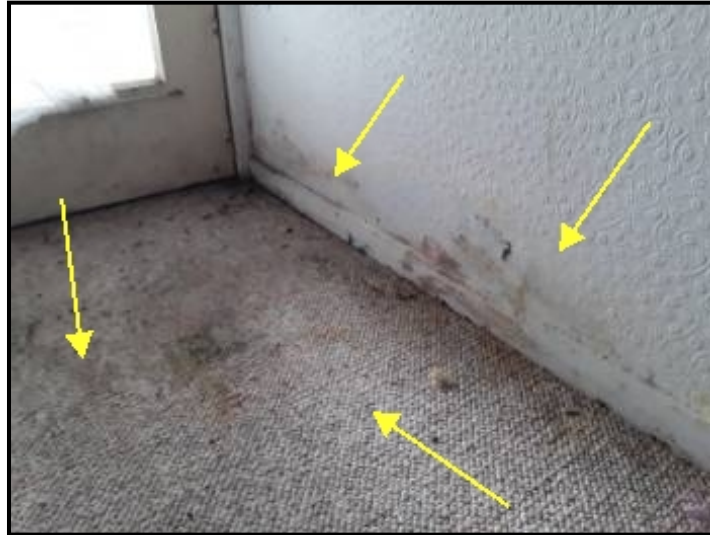
High moisture readings.
