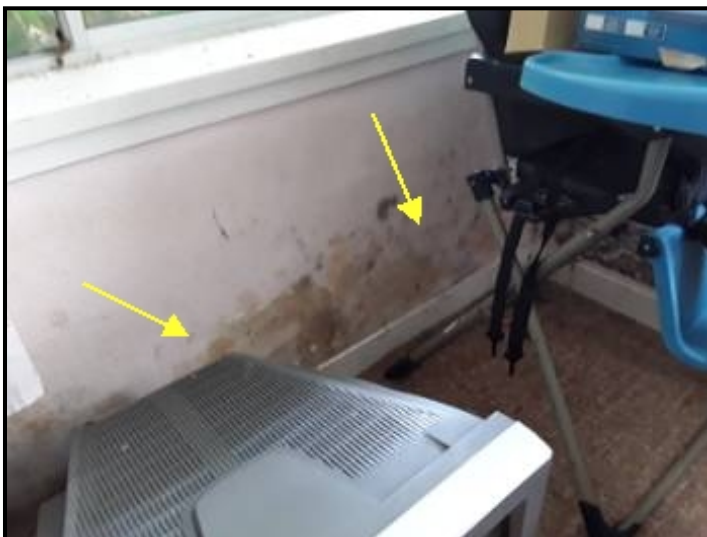
Water issues here.
