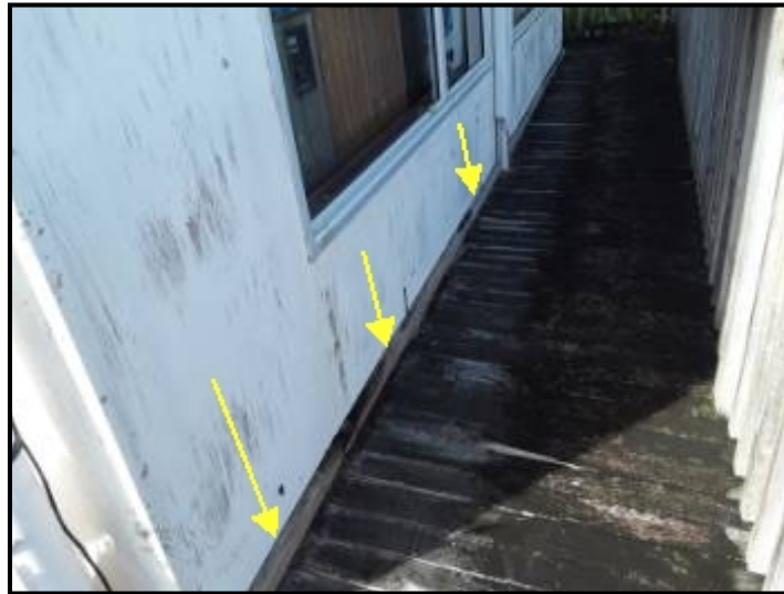
Cladding needs resealing. Ply will rot under this board.
