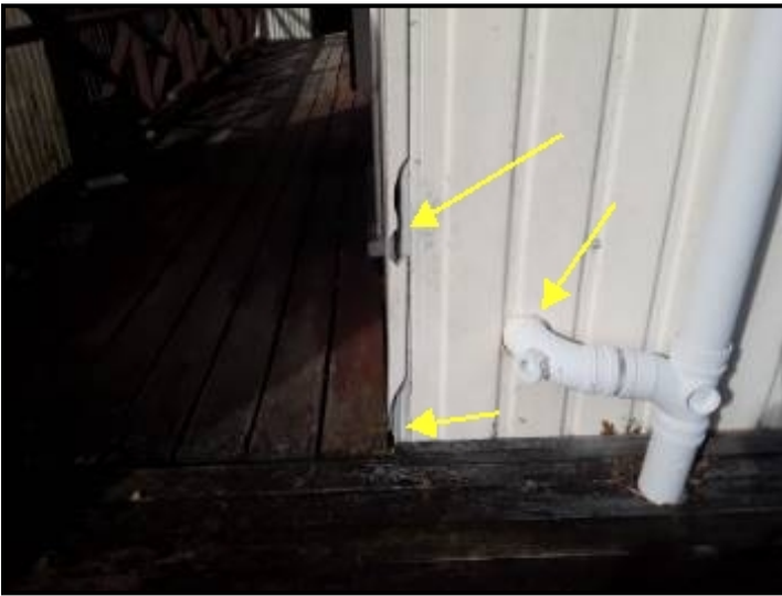
Water can seep in here.
