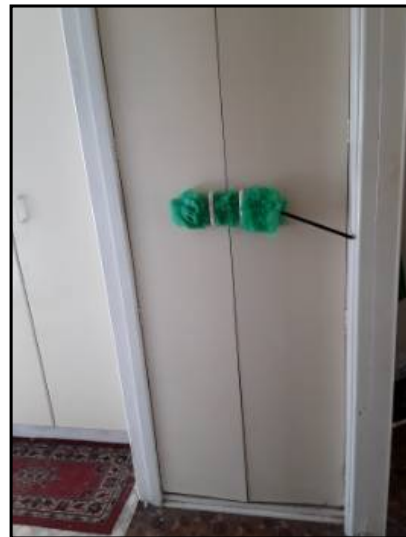
Novel door catch to hot water cupboard.
