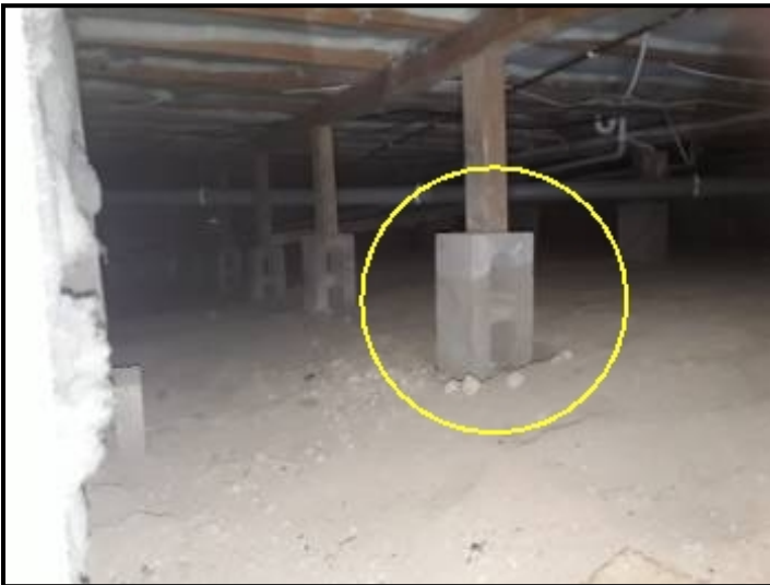
Posts incorrectly supported.
