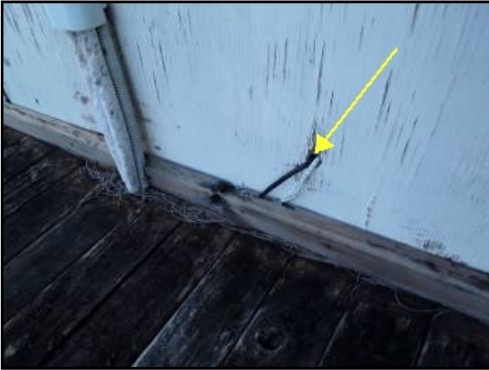
No sealant here.
