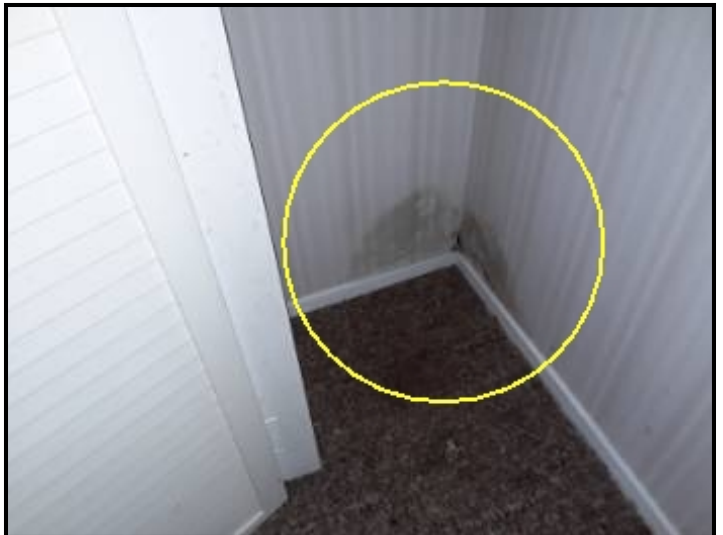
Water damage here.
