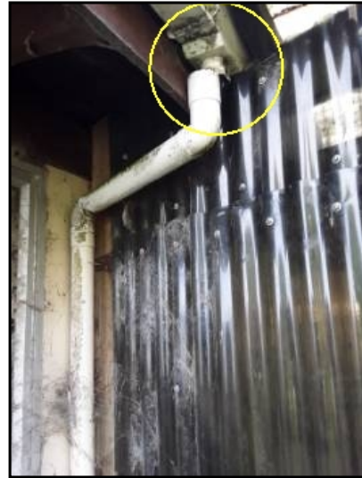
Downpipe not connected.
