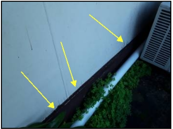
Ply rotting creating damp interior.
