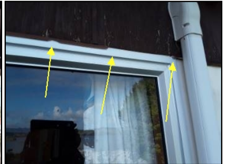
Broken head flashing.
