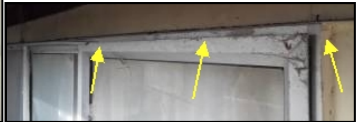
Head flashing broken.
