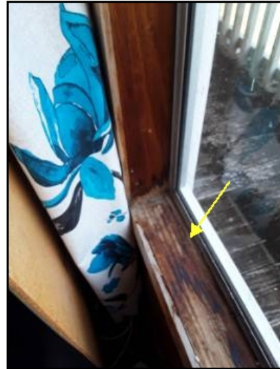
Water staining from dampness.
