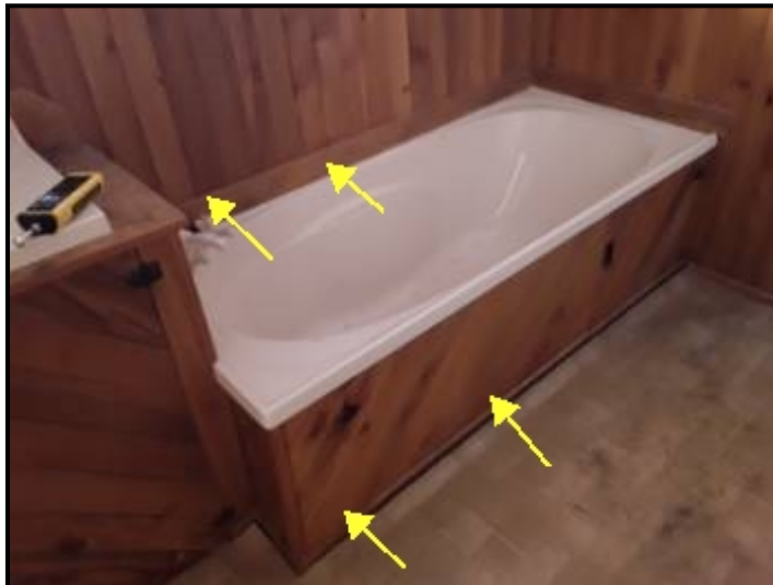
High moisture readings here.
