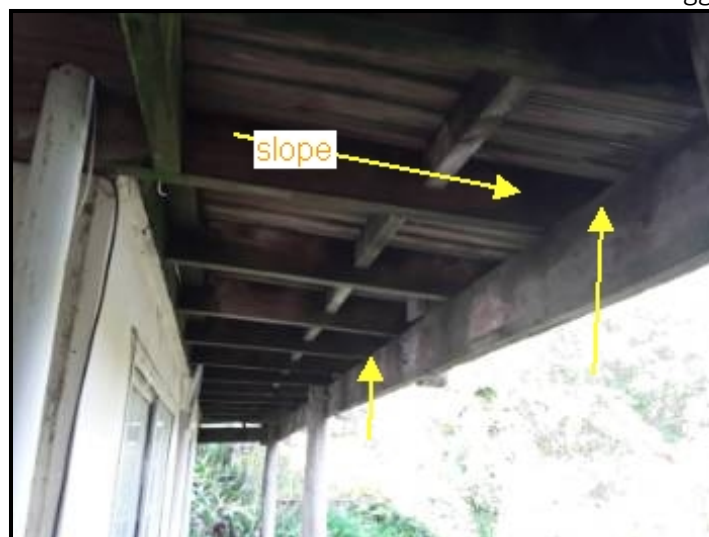
Deck joists all sloping. Suggest packing above beam.
