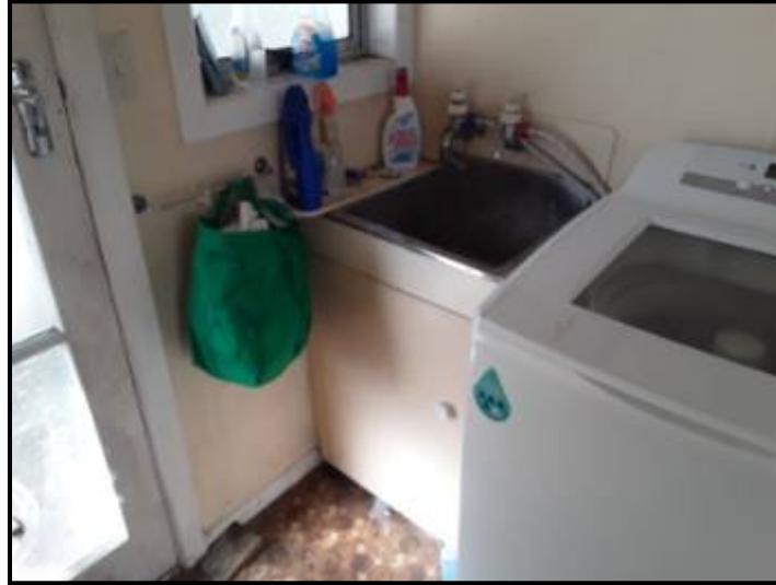
High moisture readings behind tub.
