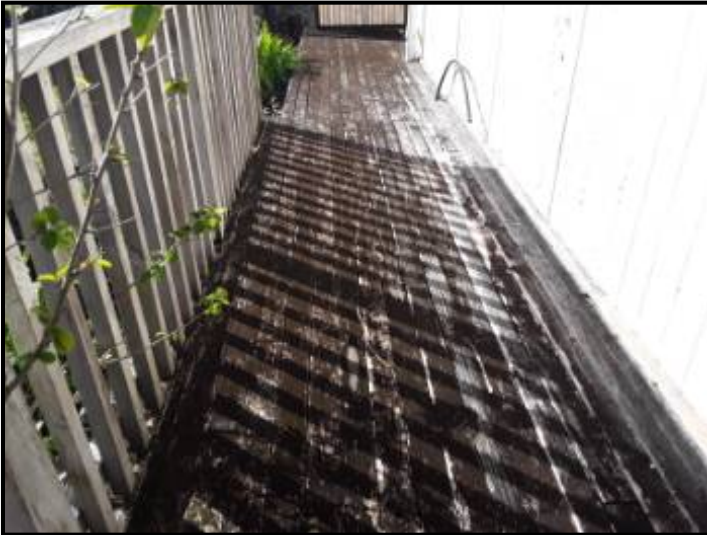
Decks need water-blast.
