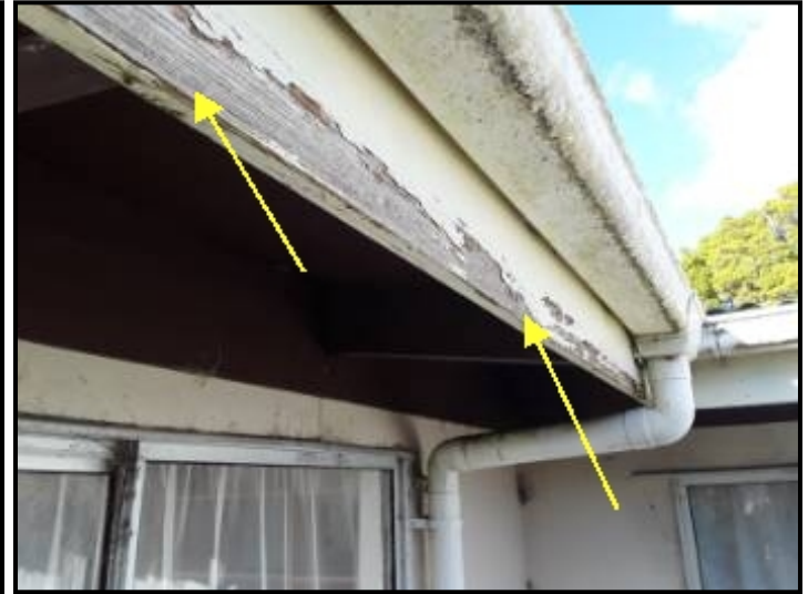
Fascias need resealing.
