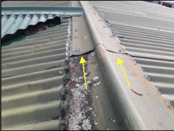
Ridge cap not sealed.
