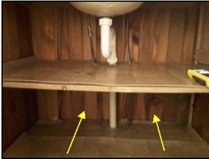
High moisture readings here.
