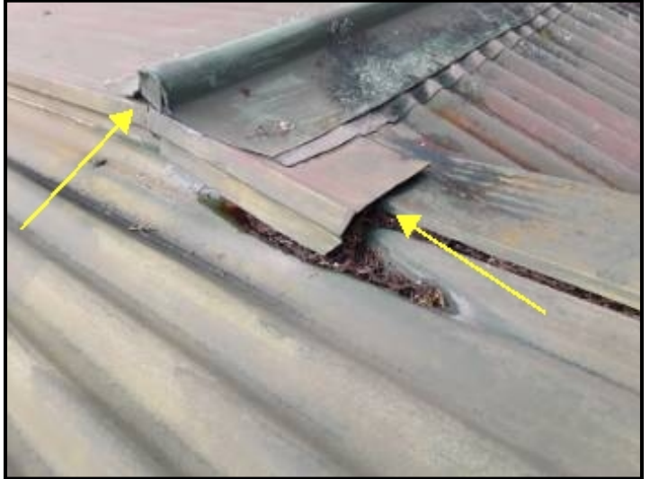
Water can drive in here.
