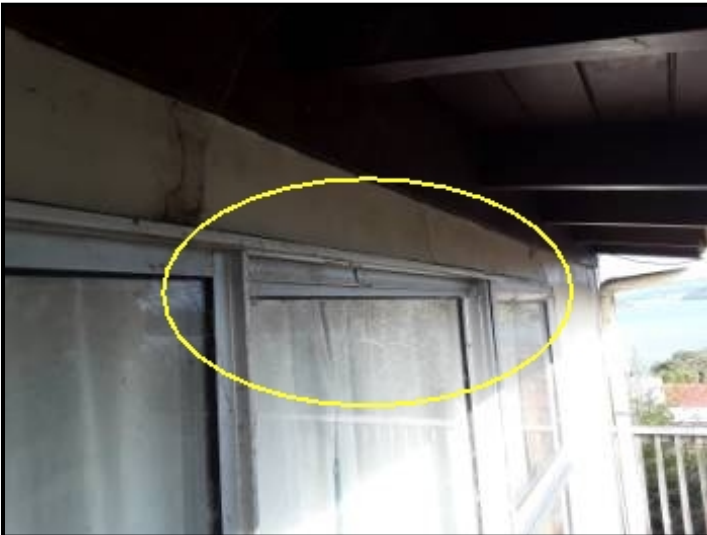
Head flashing broken.
