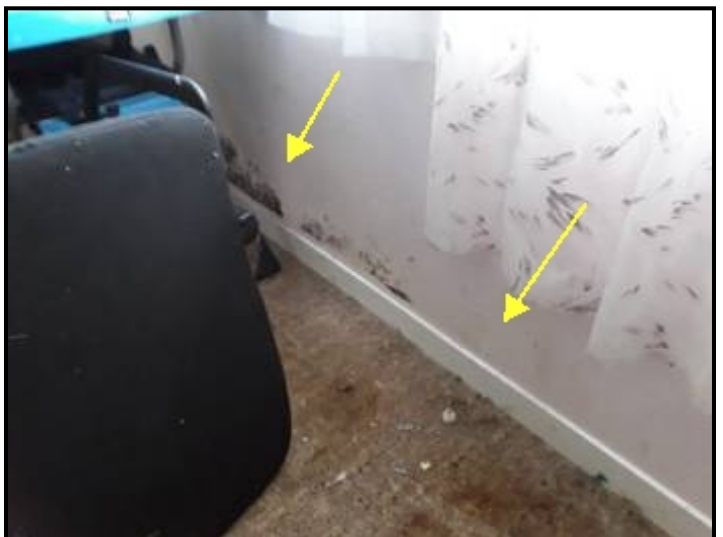
High moisture readings.
