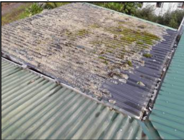
Clearlight roof needs attention.
