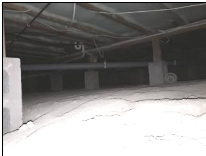
Plumbing pipes well supported.
