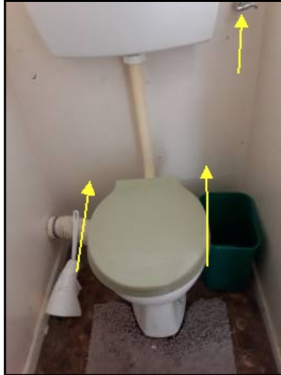
High moisture readings here.
