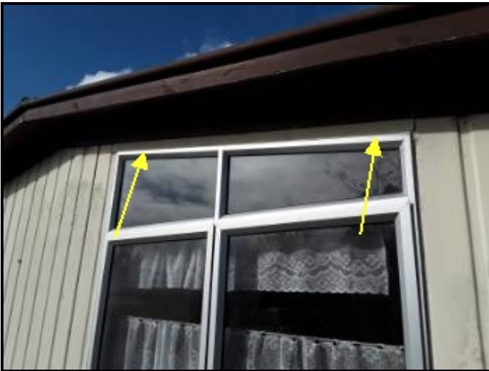
No head flashing to this window.
