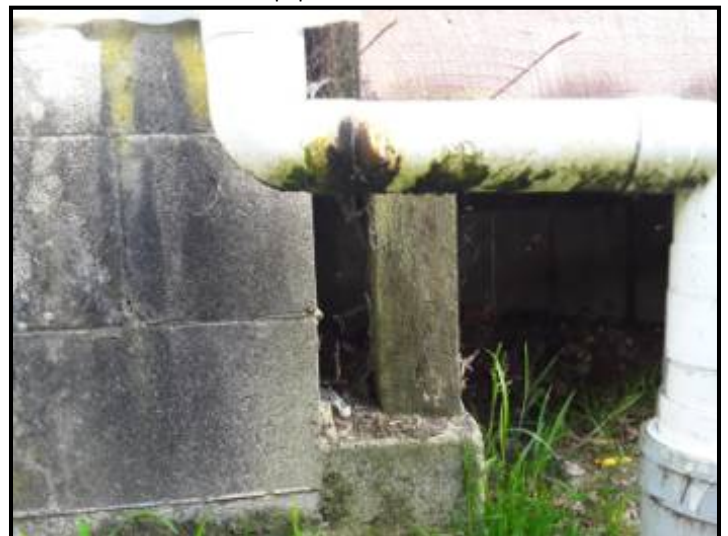
Downpipe holding water.
