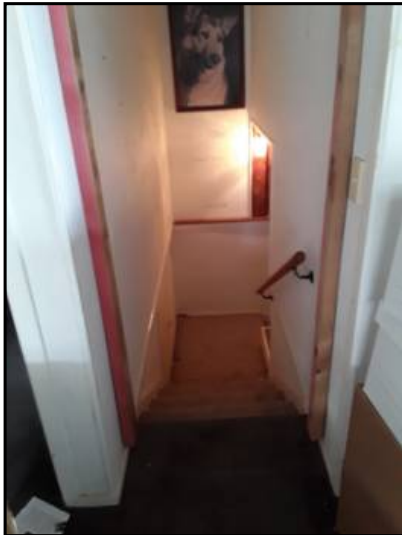
Handrail was secured correctly.
