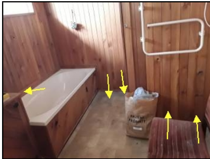
High moisture readings here.
