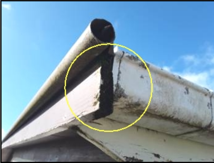
Barge board deteriorating.
