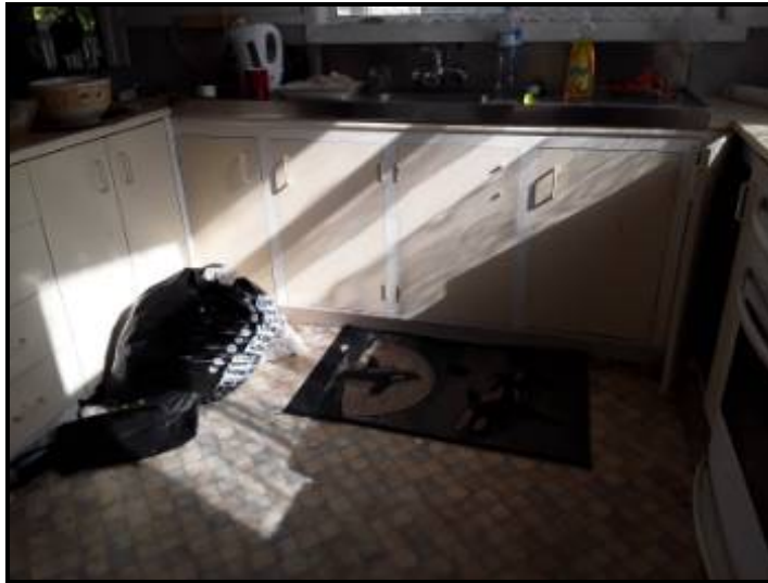
Cabinets need attention.
