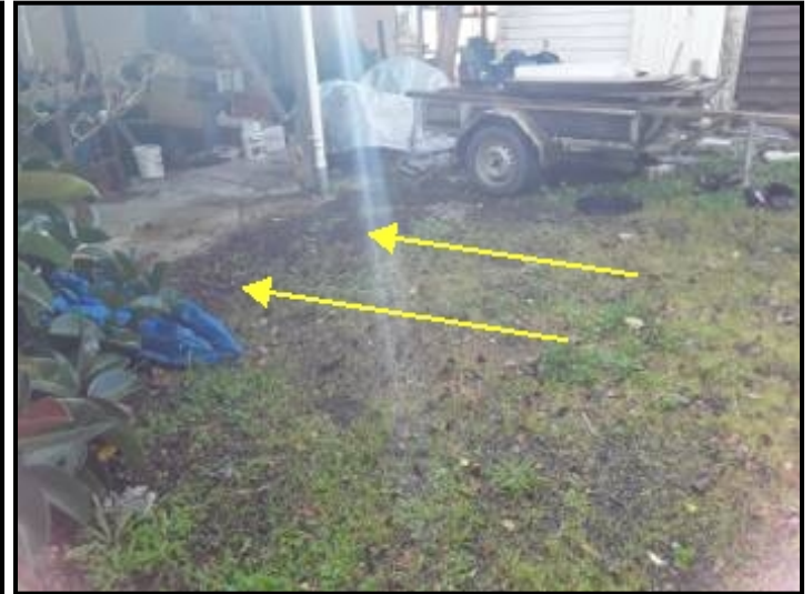
Ground slopes toward house.
