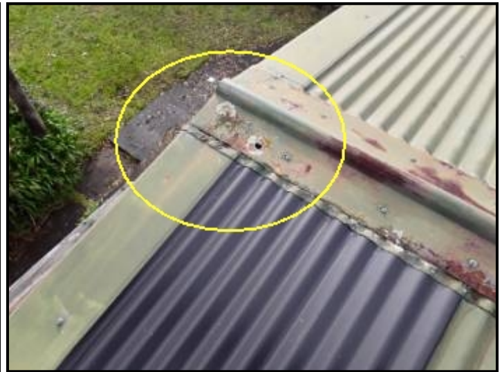
Ridge flashing holes
