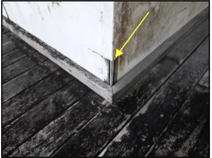
Corner flashing broken.
