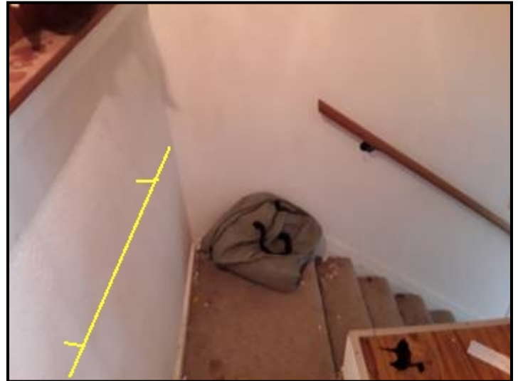
Handrail required here.
