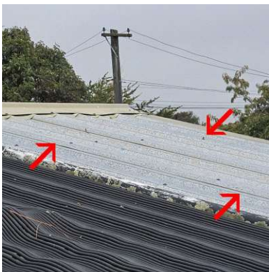
Paint peeling / Loose fixings
