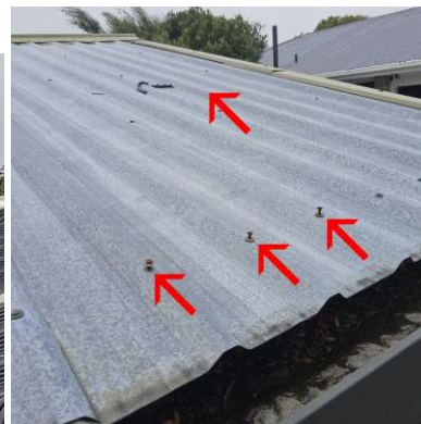
Paint peeling / Loose fixings
