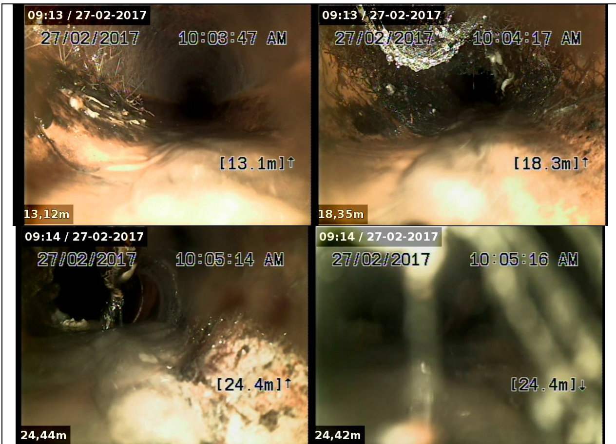
Lateral defects: joint fault, root intrusion, infiltration, blockage
