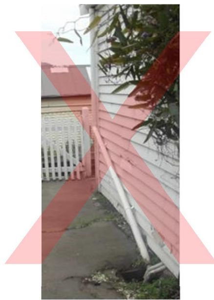
Gutter downpipe defect to low lying gully trap that allows rainwater inflow.
