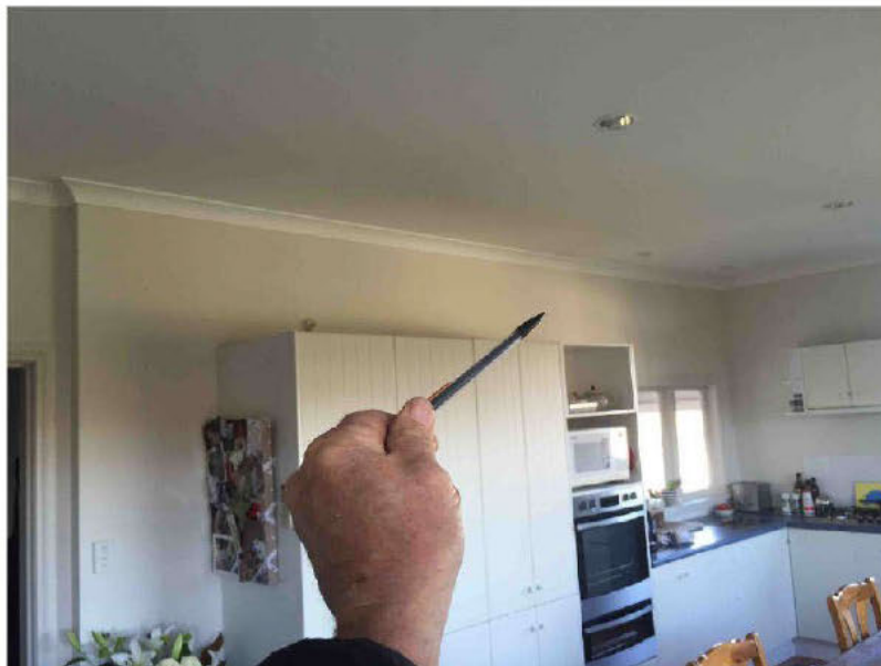
Figure 3 : Pointing to wall sheet join cracking in the kitchen
