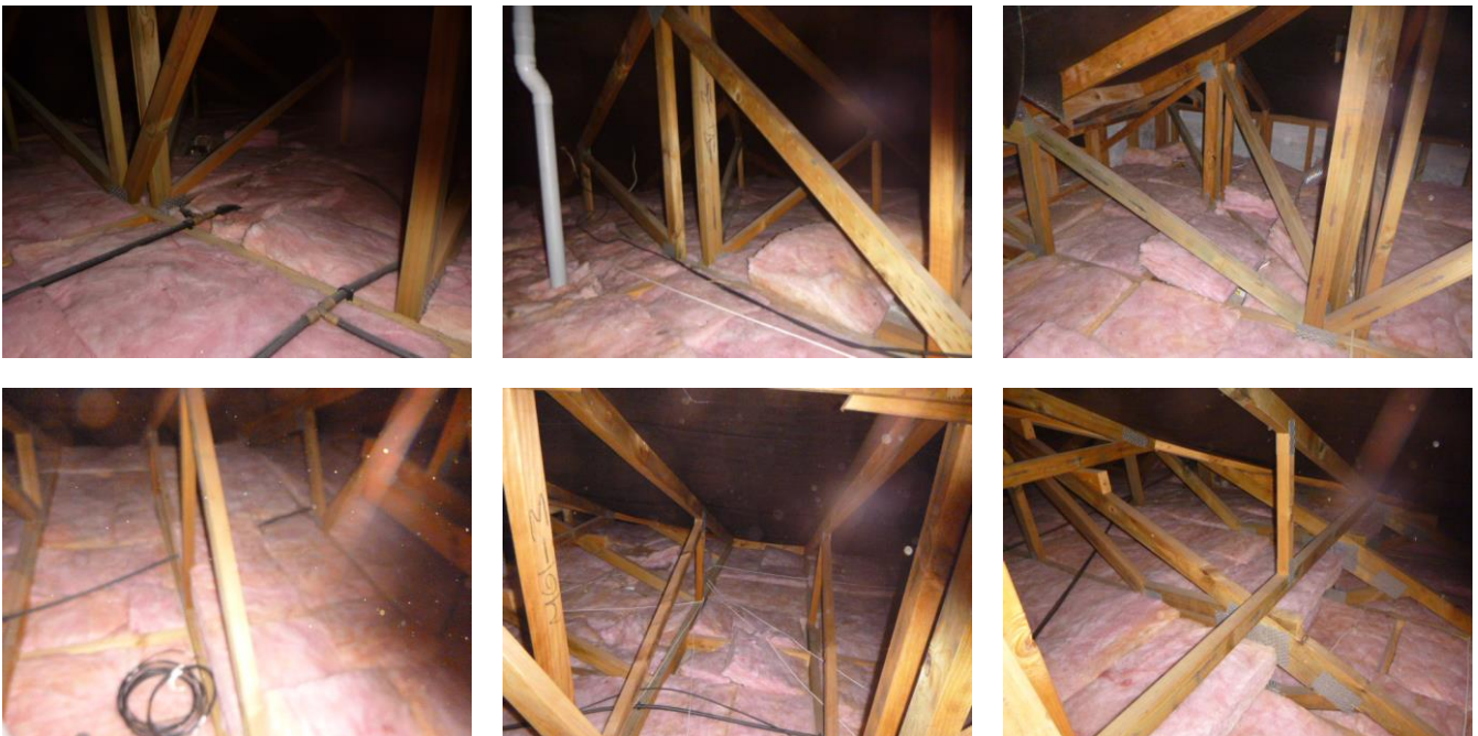
The roof cavity was dry and insulated on the day of our inspection
