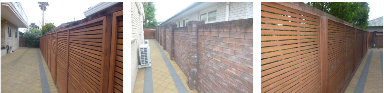
On the day of our inspection there were no signs of any excessive movement to these fences
