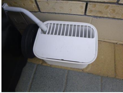
The gully trap has been installed at the correct height above the ground to prevent surface water entry
