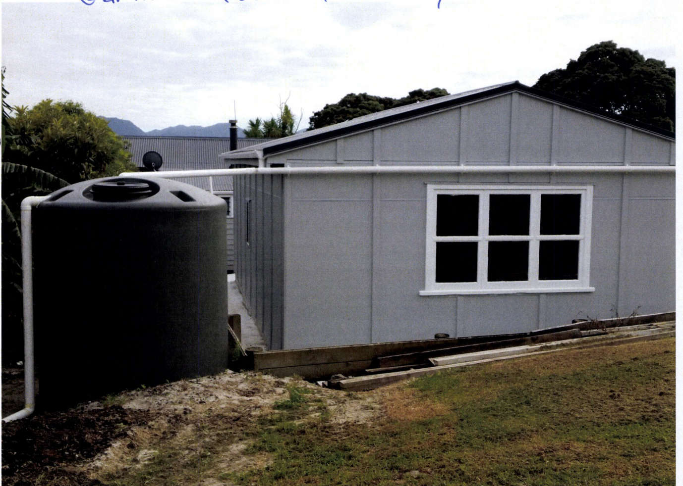
SPOUTING & DOWN PIPES & WATER TANK INSTALLED
