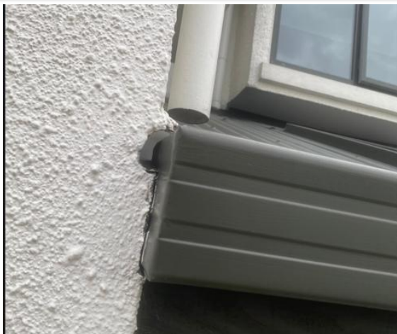
No deflector where fascia intercepts cladding
