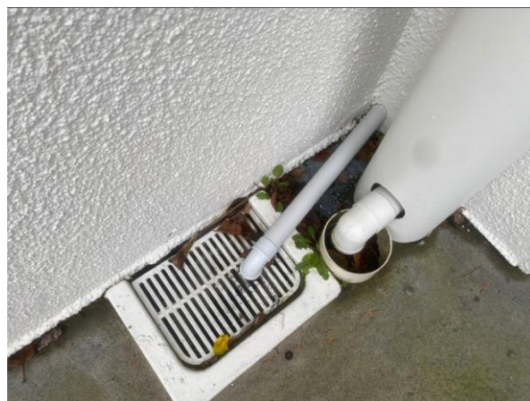
Gully trap not sealed at back
