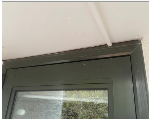
Gap above external door to garage
