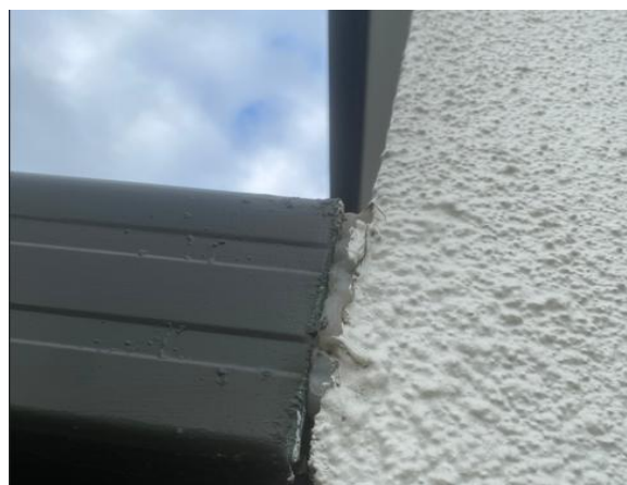
Silicone sealant in lieu of deflector flashing
