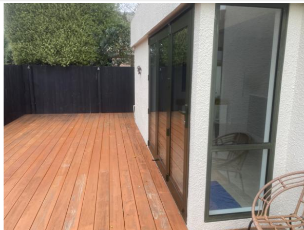
Smaller than required gap here
