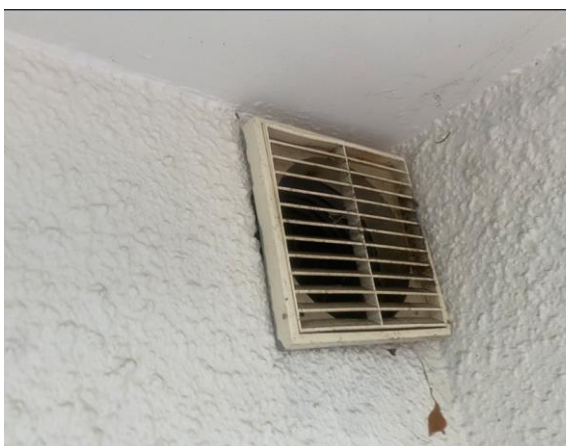
Ensure penetrations are sealed
